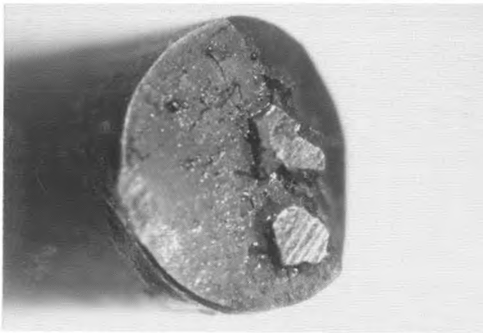
Figure 5.31. Outer wire failure 3 to 6 inches from bearing face of top anchorhead, strand 10
