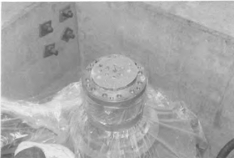
Figure 5.21. Grout cap removed; break occurred at top of strand extensions
